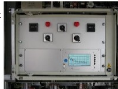
SPECmonitor in a hJ619* rack
