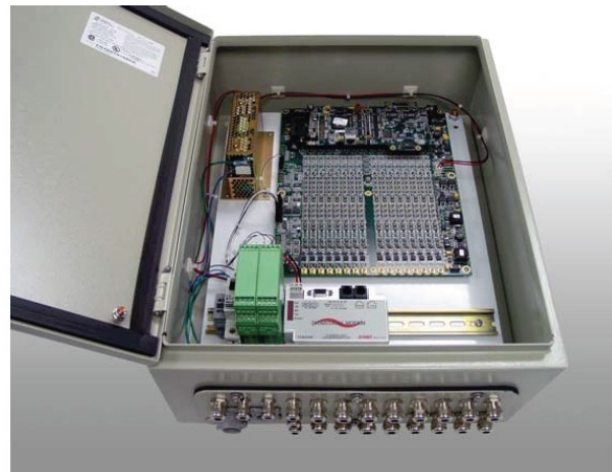
Figure 1. Inside the Sensor Highway Cabinet
