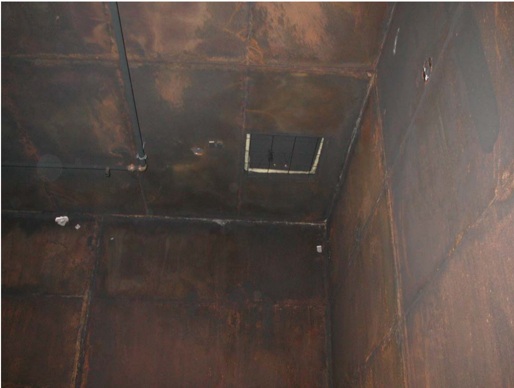
Photo B3 One (of the two) small over pressure vents at the ceiling.
