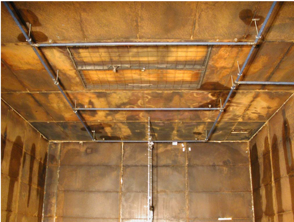
Photo B2 The pipe-work for the water spray and low-pressure water mist system. At the centre of the ceiling, the steel hatches for the large ventilation opening.
