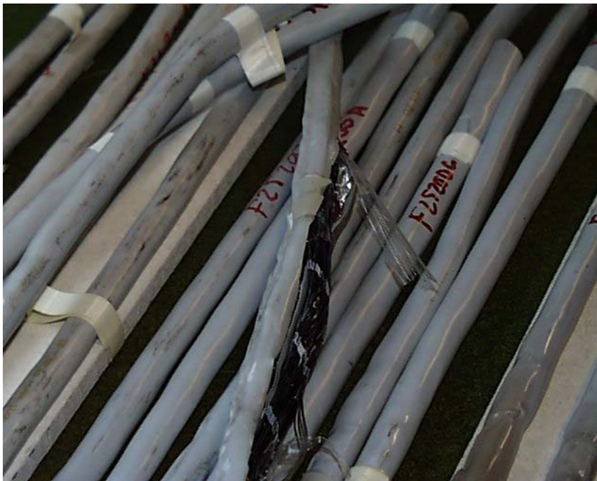
Figure A2-8. Cables after the test. One of the cables has been cut open to see how damaged the cable is on the inside. As seen the cables are not very damaged on the outside.
