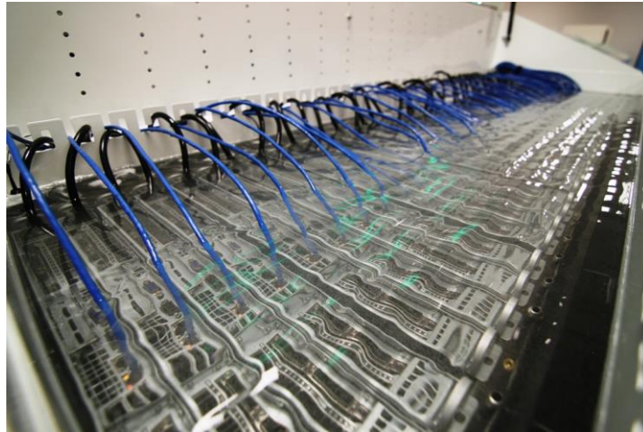
Figure 34: Immersed servers in a non-conducting dielectric fluid.
