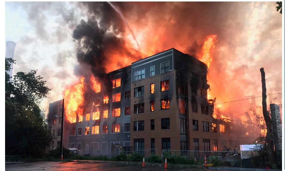
Figure 3.10 Fire in Timber Frame Apartment Building Under Construction (Source: Captain John Bonadio, Waltham Fire Department, as published at https://www.enr.com/articles/42484-what-local-officials-want-to-do-about-wood-frame-building-fires-in-massachusetts ), Courtesy of Waltham, Massachusetts Fire Department)
