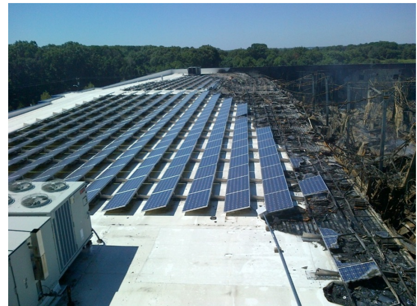
Figure 3.9 Aftermath of Delanco, NJ, Warehouse Fire (Courtesy of New Jersey State Fire Marshal Office)
