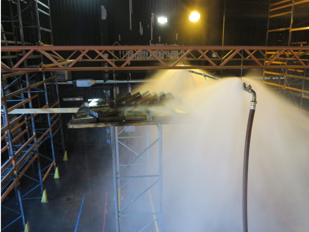
Figure 6 Test 1.4: The water spray pattern of the Tyco model EC-25 sprinkler at the maximum pressure of 4.2 bar obtained with the pump. The water flow rate per sprinkler was 760 liter/min.
