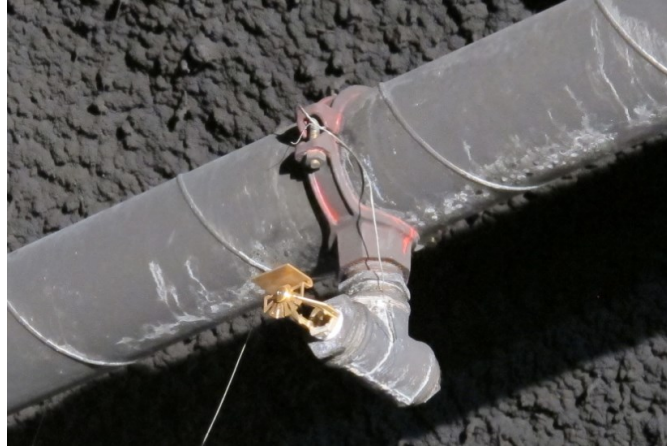
Figure 5 The nozzles were fitted with a T-coupling to a pipe with a diameter of 140 mm, located at the ceiling and close to the tunnel wall. The nozzles were mounted every 5 m, and sprayed water horizontally in one direction [6].
