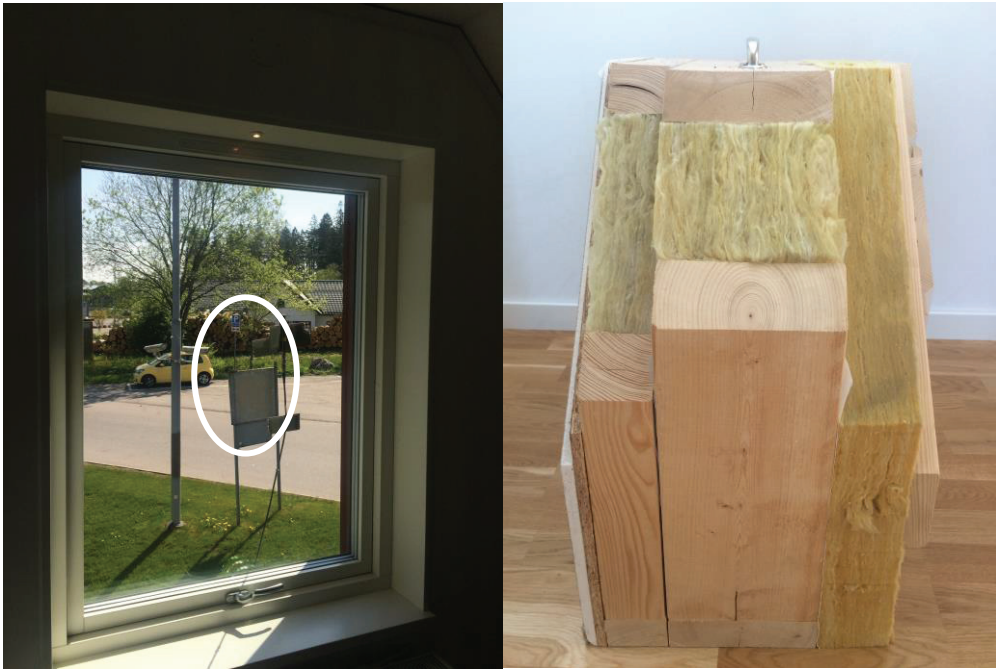
Figure 3 – The microphone was attached to the window with adhesive tape (left). The construction details and individual elements are well documented. The picture to the right shows a cross-section of the façade.
