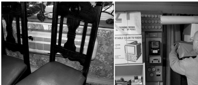
Figure 3a: A hidden air pump. Figure 3b: An electricity meter uncovered in the basement.
