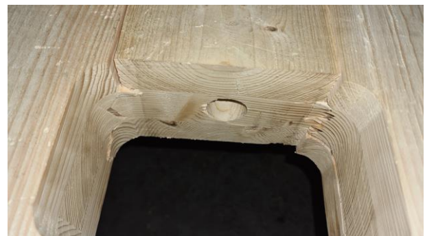
Figure 11: Test 1 local damage under the washer
