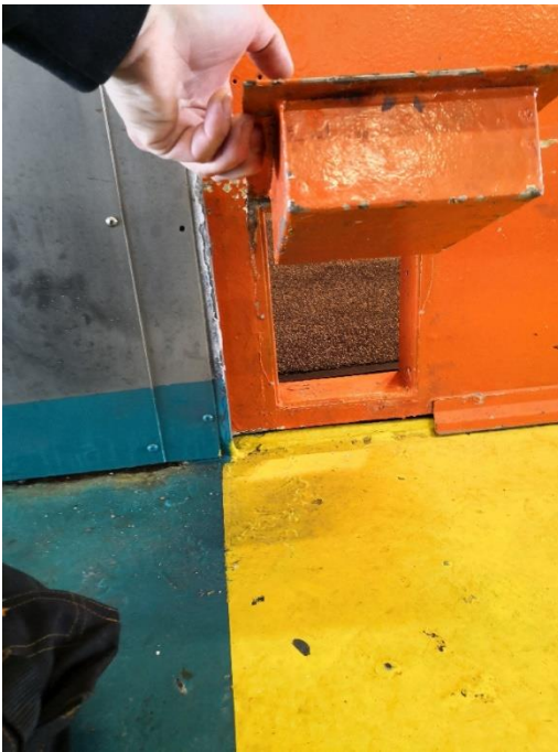
Figure 7 Example of “cat hole” in sliding door
