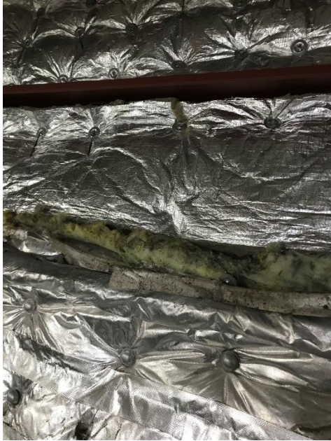
Figure 4 Example of damaged fire insulation
